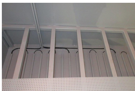
The GeoBag™ units can be isolated and heated for areas with colder climates.
